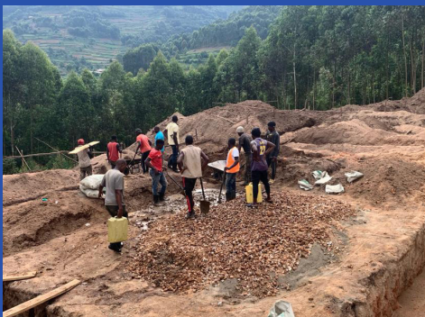
Work has already begun at the new Hope High School campus in Rubanda
